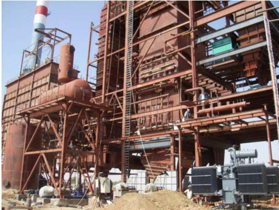
Figure 68. Transtech Green Power Ltd. has set up a 12 MWe biomass power plant in Sanchore in Rajasthan state (Tandon 2014).
