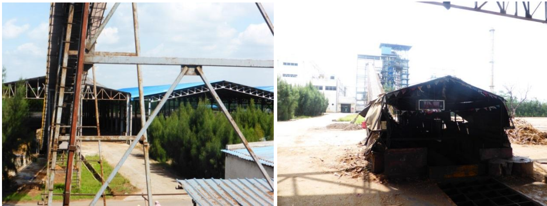
Figure 58. The conveyor feeding biomass to the boiler (Photos by Arvo Leinonen).
