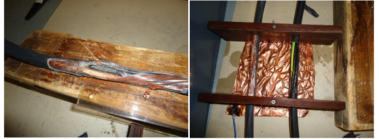
Fig.2 Cable sheath removed from the AMCMK cable (left). Both cables installed at a container (right).
