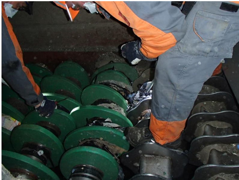
Figure 31. Cleaning of the recycled fuel screen at the power plant C.
