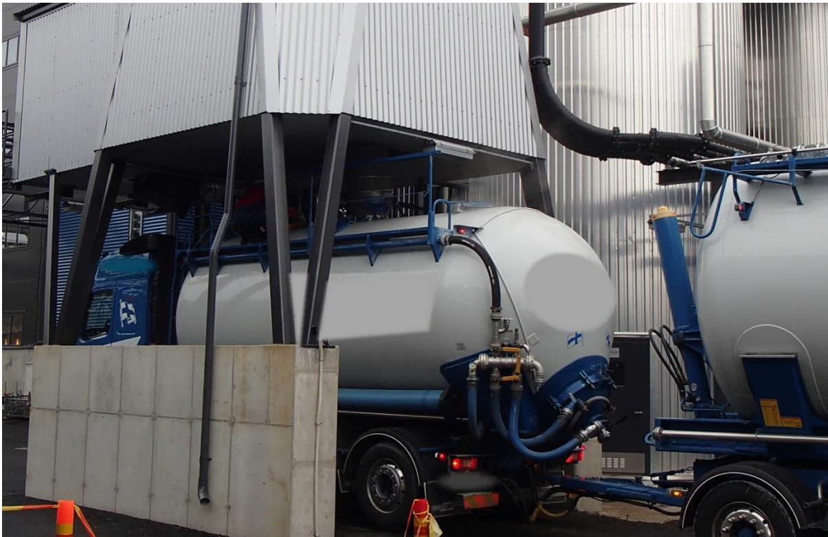
Figure 7. Loading of dry fly ash to a tank truck.
