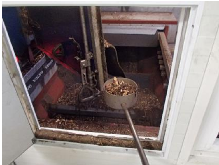
Figure 60. Fuel sampling from control room.
