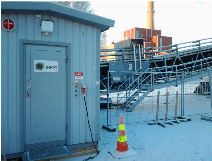
Picture 1. Inray Fuel at UPM Kaipola power plant at the end of beginning of the fuel conveyor
