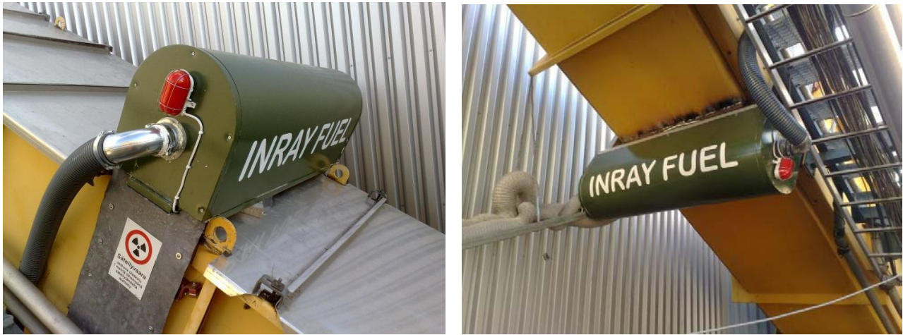
Image 15. The radiation source unit and the detector unit of the X-ray based Inray Fuel mounted in a conveyor of a power plant.
