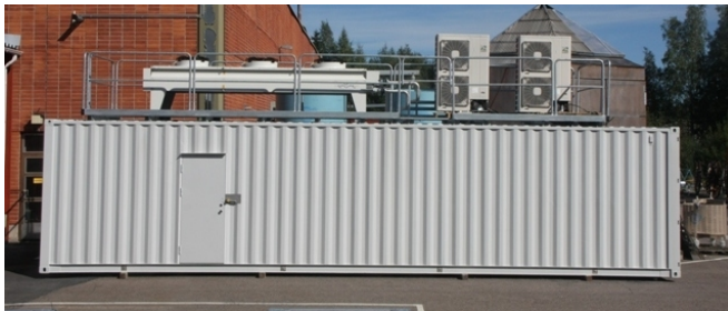
Figure 4: STATCOM in a container
