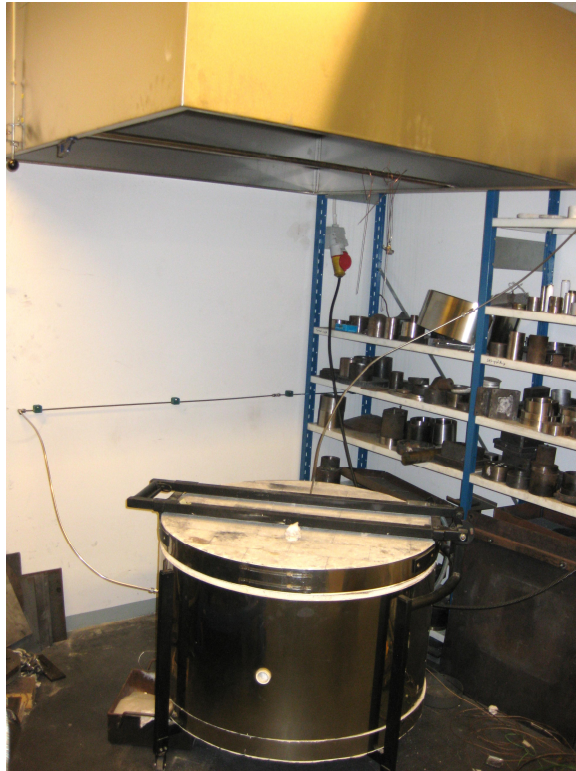
Figure 6. The furnace in operating position. Gas outlet comes out from an opening of the furnace lid. Ventilation hood connected to powered roof ventilation ensures gas evacuation in the case of mall function. Methane alarm system will be installed before oxygen carrier testing work.
