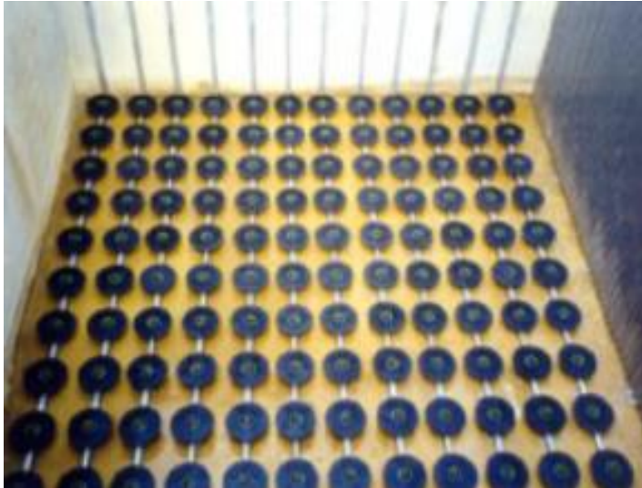
Figure 5. Membrane disc diffusers in wastewater treatment plant.
