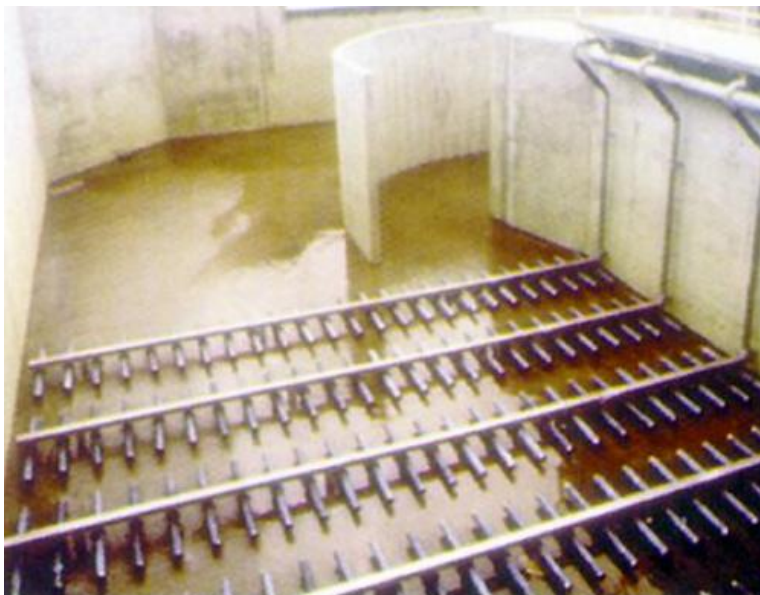
Figure 6. Membrane diffusers in wastewater treatment plant.
