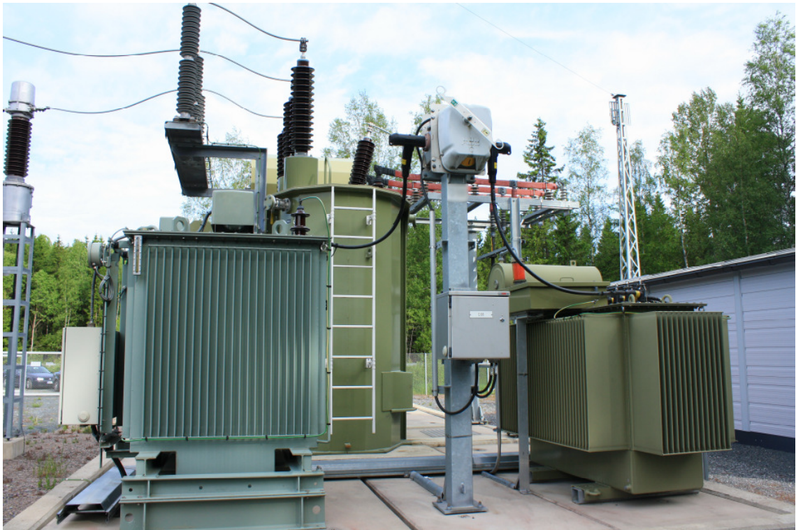
Figure 4.3 An earthing transformer (left) and the Petersen coil (right). Between the neutral point devices a disconnector.
