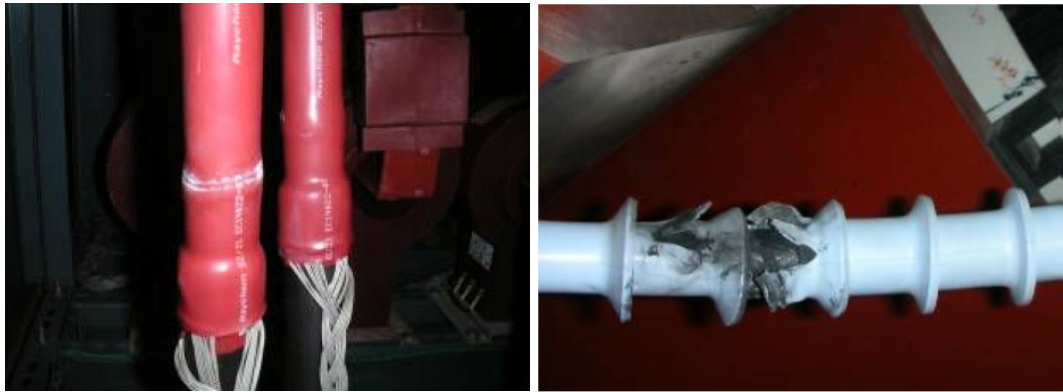
Figure 3.8. Surface discharge ring on top of termination probably due humidity and dirt (left) and high impedance fault in termination (right) [25]
