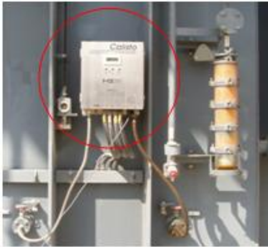
Figure 6.8 On-line dissolved gas monitor connected to a transformer
