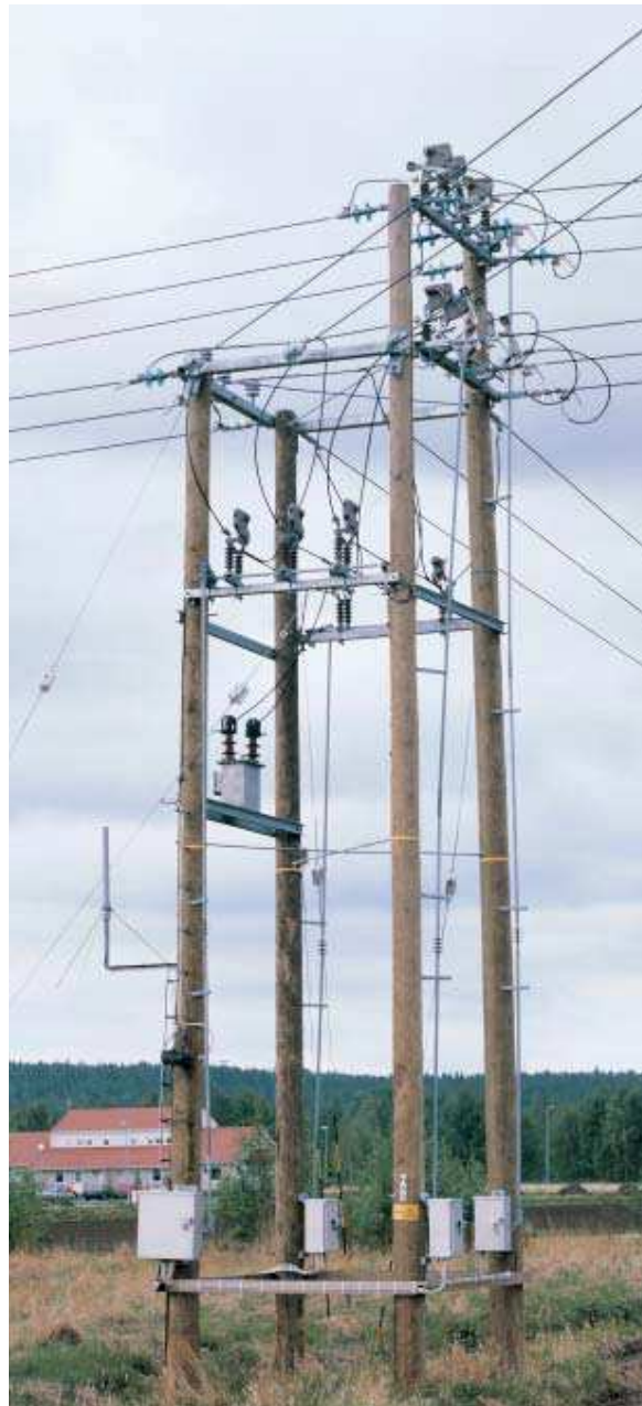
Fig. 5.2. Remote controlled pole mounted disconnectors station, Foto ABB
