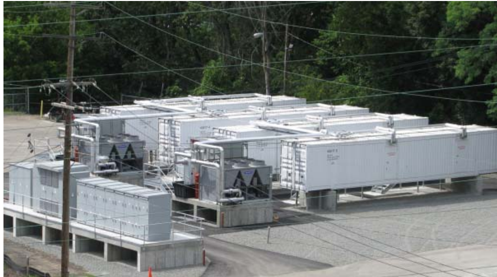
Figure 5-19. 8 MW Lithium-ion battery system in Johnson City, N.Y. [Source: AES Energy storage].
