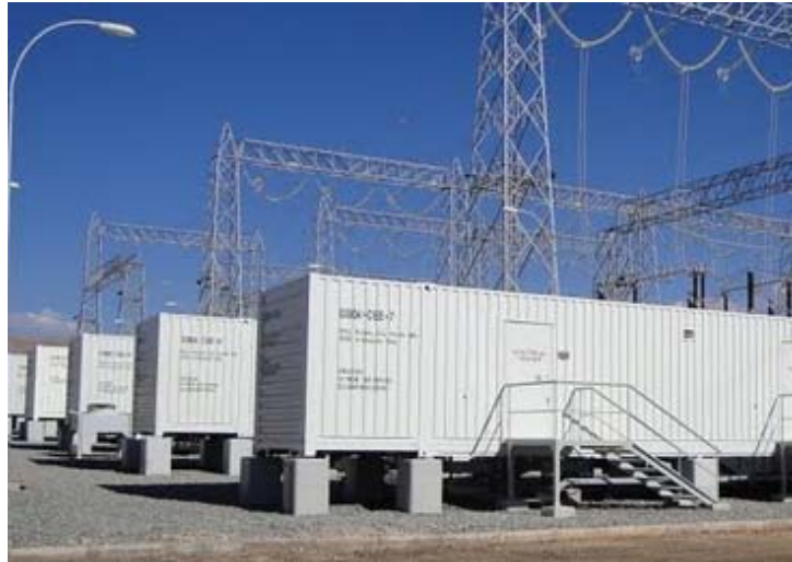
Figure 5-20. 20 MW Lithium-ion battery system for spinning reserve in Chile [Source: A123 systems].
