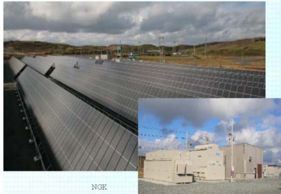
Figure 5-44. An example of ES installation for solar farm integration [Source: NGK].
