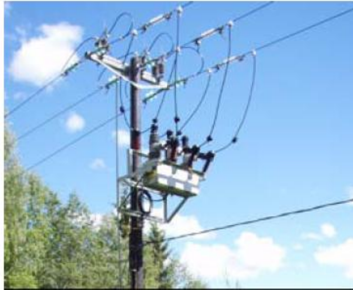
Figure 9. An example of a MV feeder with a recloser (ABB picture).
