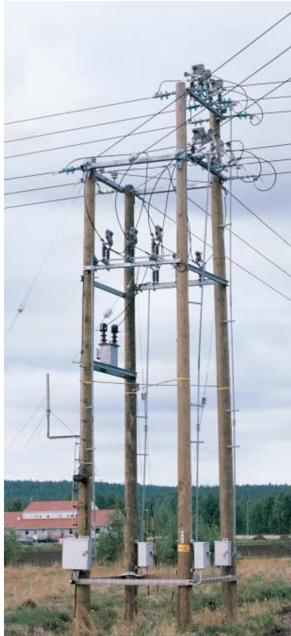
Figure 10. An example of a MV feeder with a disconnector (ABB picture).
